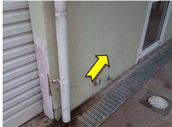
Photo 8. Exterior, throughout, walls – suspected lead-containing light green upper paint system.
