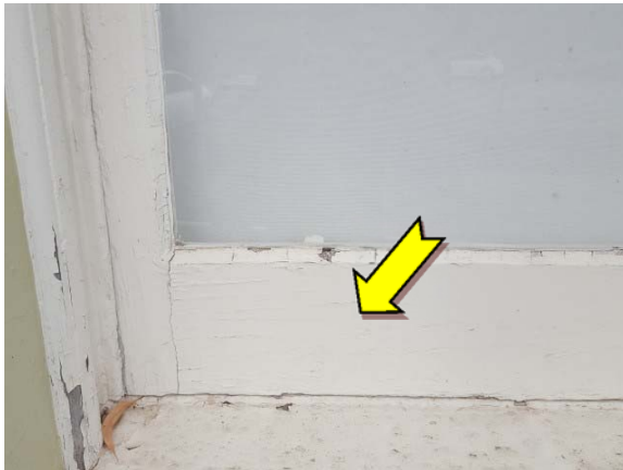
Photo 9. Exterior, throughout, window frames – suspected lead-containing white upper paint system.
