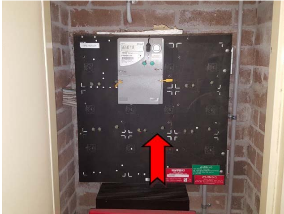
Photo 1. Interior, ground level, store room, electrical board – suspected asbestos-containing bituminous backing board.
